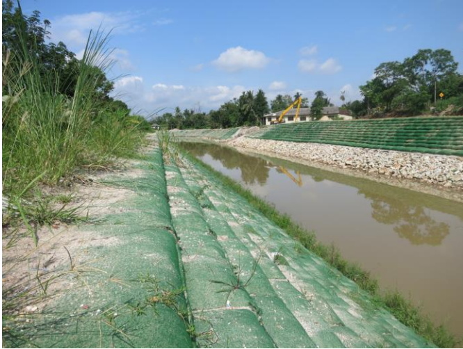
Supply at Sungai Rasau - 2016
