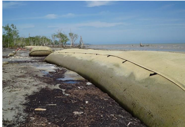
Supply at Pantai Kelanang, Selangor -2016
